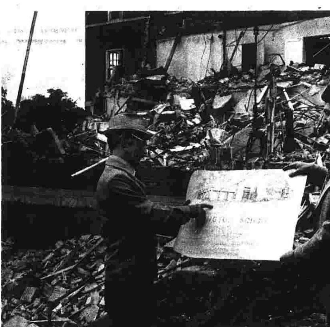
Making plans as wrecking starts With the wrecking process of the West Side Recreation Center on Cedar St. going on in the background, Paul Phillips, town building committee chairman, and Arnold Lawrence Jr., architect, study the plans of the new recreation building that will be constructed at the same site. The wrecking began today. (Herald photo by Pinto)
